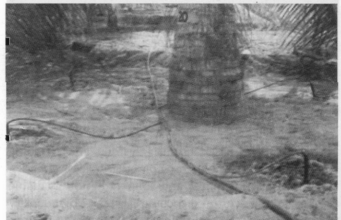
Drip irrigation system
