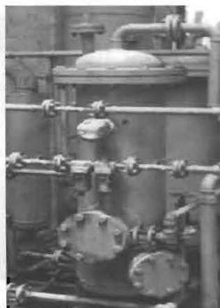
Fig. 5 Nitrogen Purging Machine
