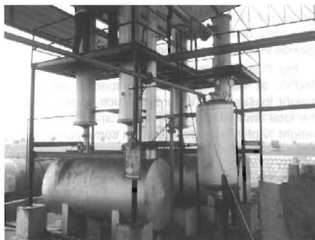
Fig. 3 Bio-oil Condensers and Oil Collectors
