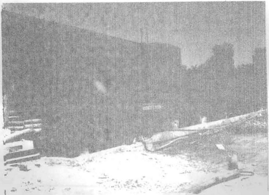
Fig. 4. The expensive and sophisticated vacuum/pressure treatment plant. (Courtesy of Davao Woods Preserving Company, Inc.)
