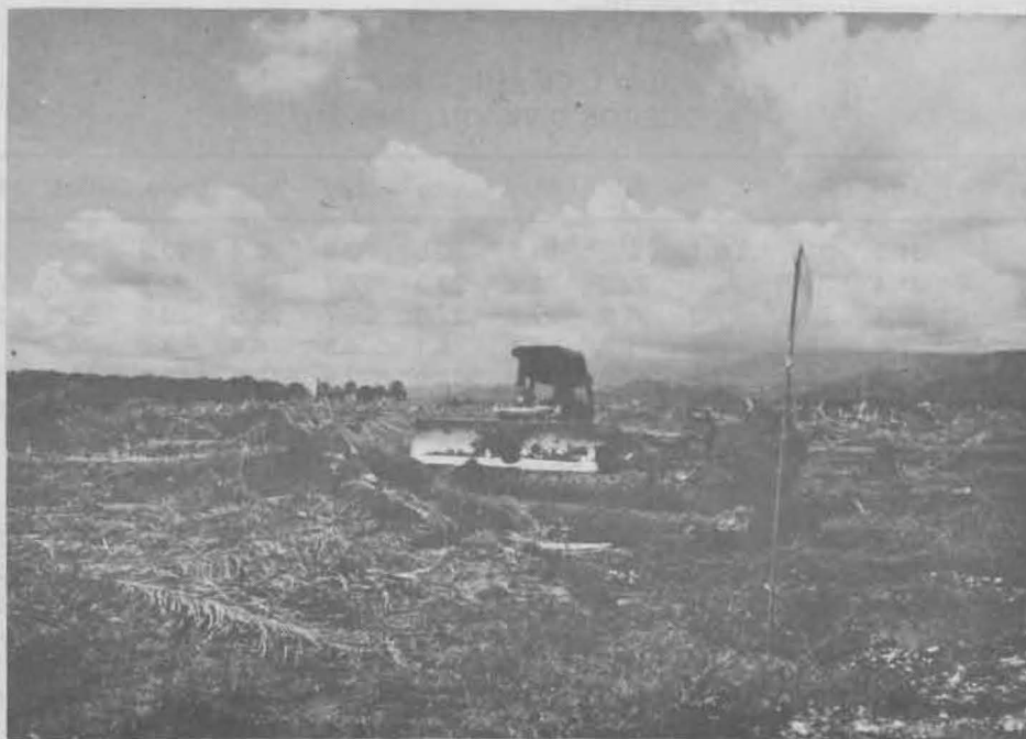
Piling of cut Palm trees using a bull-dozer for burning and replanting
